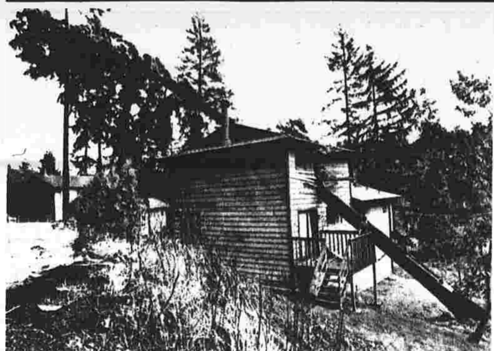
Terry Dunn stands on the deck of his home in Seattle, Wash., viewing the damage done by strong wind gusts which toppled a towering fir tree through his roof shortly after dawn Thursday. A wild storm swept
